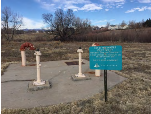
Photo 1. Looking west at the northern terminus of the BDCIS project. Note the sign reads “City of Westminster Utility Facility Interceptor Diversion Structure #1.”
