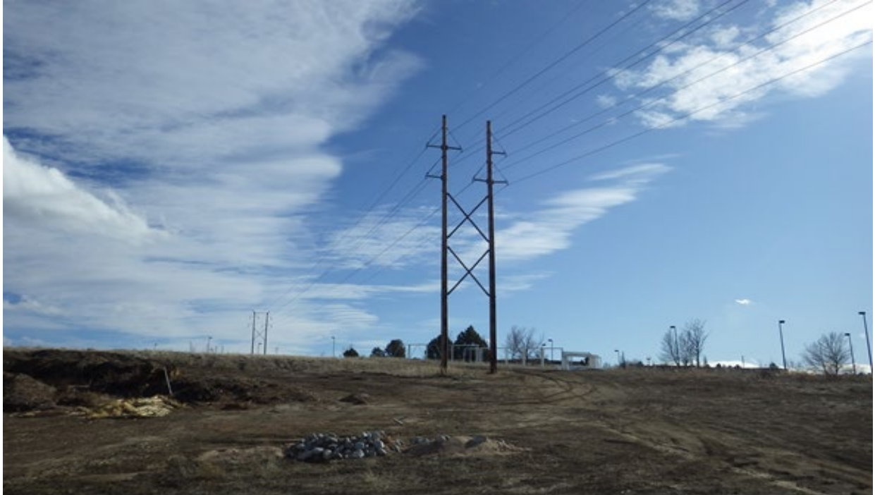
Figure 3: Xcel Transmission Line 9055 facing southeast.
