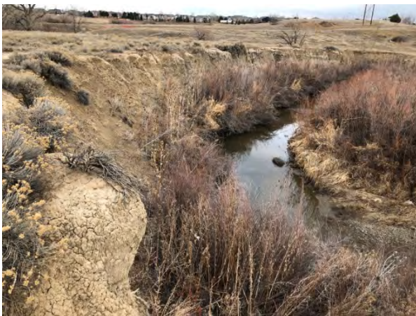
Photo 6. Looking north-northwest at stream S-1g in the middle portion of the project study area. Note the large amount of stream bank erosion and slumping occurring on the northern bank.
