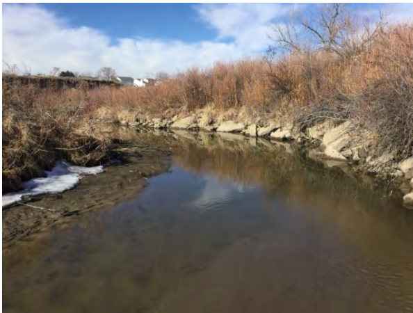
Photo 2. Looking west (upstream) at stream S-1b in the northern portion of the project study area. Note the large amounts of riprap stabilizing the northern bank of the creek.
