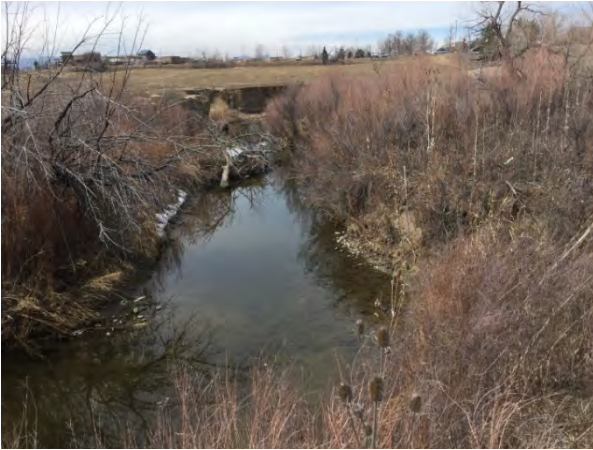
Photo 10. Looking south at stream S-1j in the southern portion of the project study area. Note the large amount of stream bank erosion and slumping occurring on the stream bank in the background.
